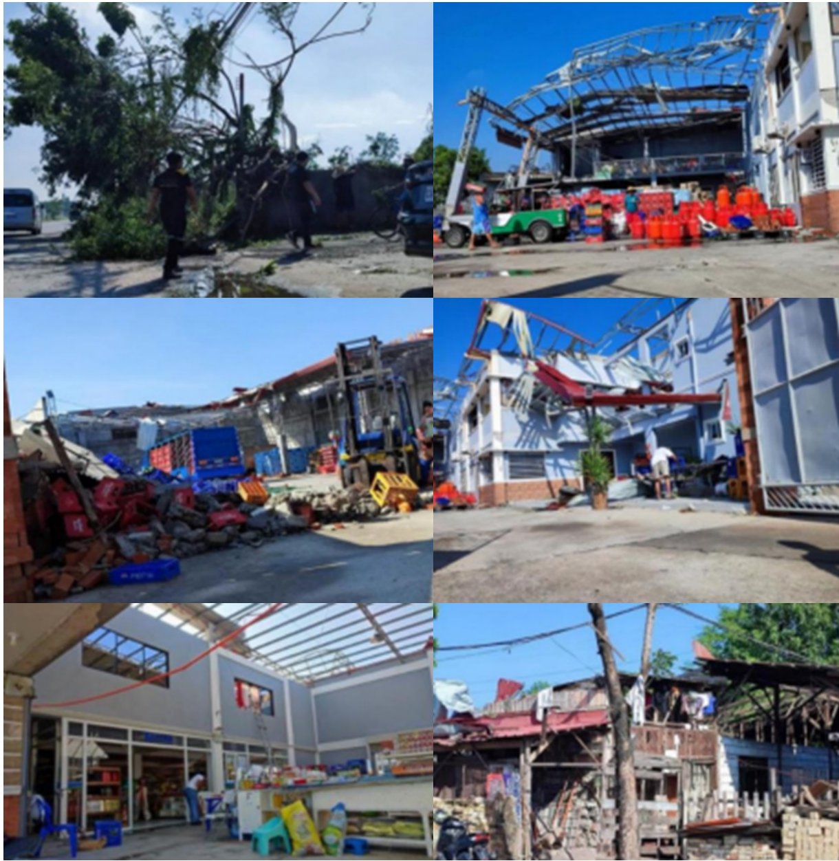
Damage infrastructure at Baytra Supermarket along San Fernando – Lubao Road, Sitio Banlic, Bacolor Pampanga. (MDRRMO Bacolor)
