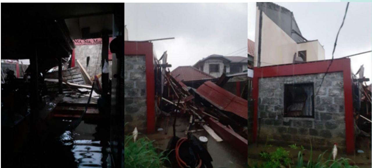
Damage properties at Pasig San Rafael, Macabebe, Pampanga after the onslaught of tornado over Pampanga. (MDRRMO, Macabebe)
