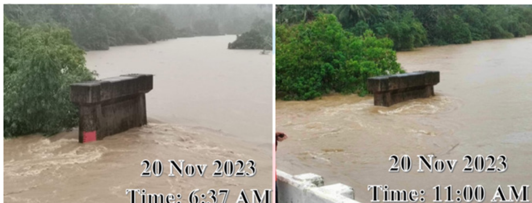
Sudden rise of the water level of Catarman River, Catarman, Northern Samar. Photos from DRRMO Catarman.
